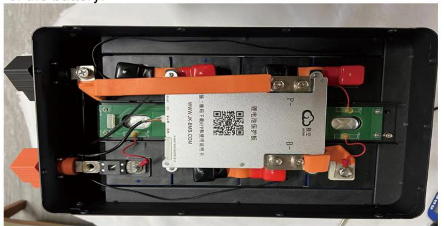
26. Take out the 250A fuse from the accessory box and connect the total positive pole of the battery and the positive output terminal.
