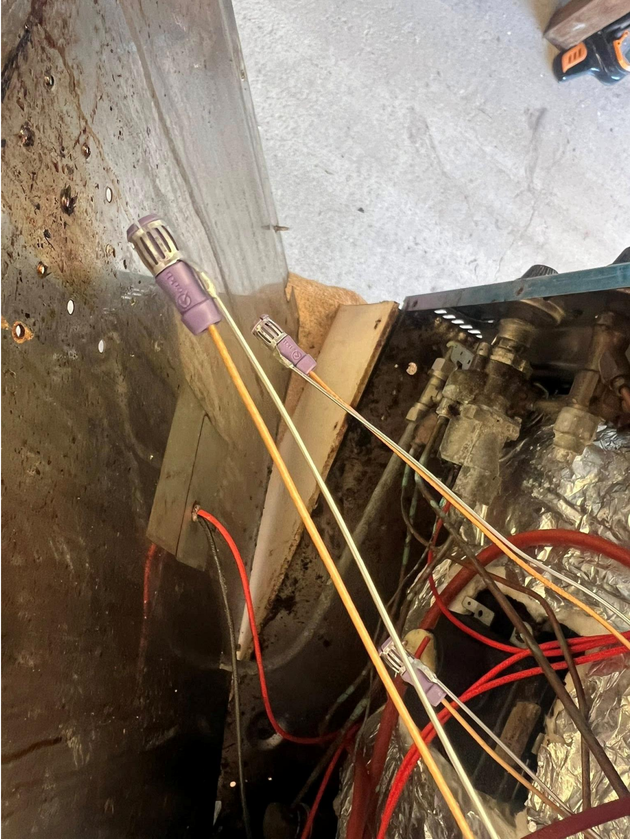
New thermocouples awaiting plugging in.
